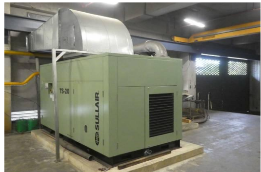
Figure 7 Air Compressor System
